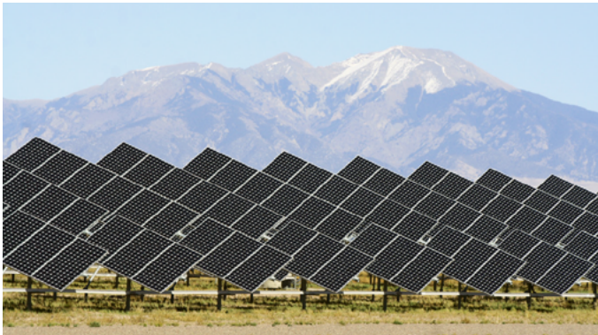
ACME screws position solar panels
